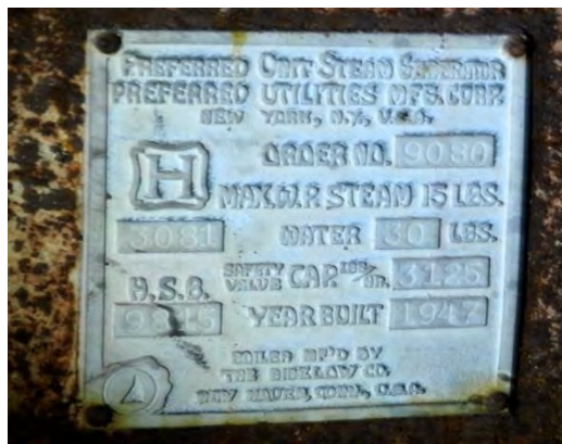
Existing boiler manufacturer by Preferred utilities
