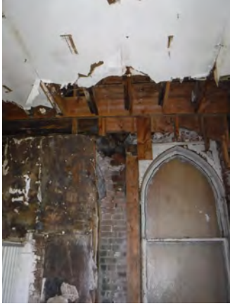
Interior damage towards roofs
